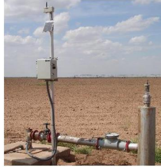
Irrigation – Water Flow and pipe pressure monitoring
